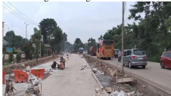
Figure 4. Photograph of Traffic Congestion at Musi II Bridge Affecting Ready-Mix Distribution
