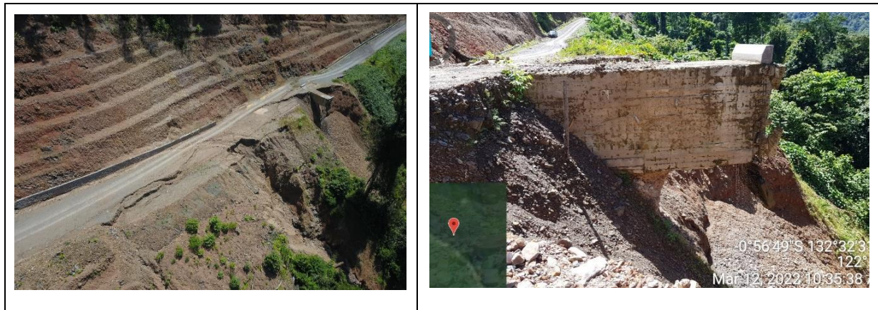
Figure 2. Road Damage Condition Due to Landslide
